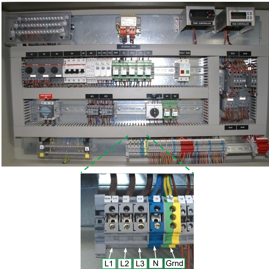
Figure 4-5. Electrical switchboard and electricity terminal block
