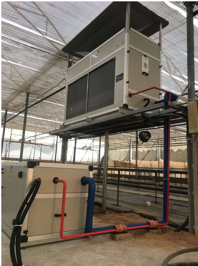
Figure 9-7. DryGair split unit
