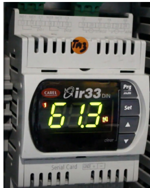
Figure 9-6. Temperature valve controller
