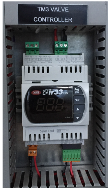
Figure 9-16. Temperature valve controller
